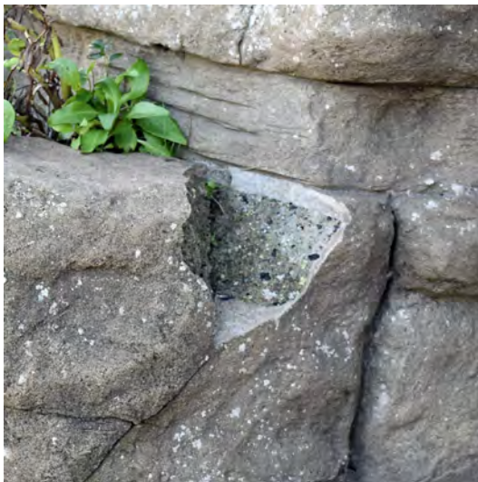
5.11: DEEP LOSS OF CONCRETE BACKING (C08) — POSSIBLY FROST DAMAGE.
