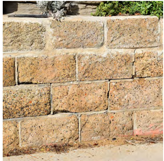
5.24: FAILED CEMENT POINTING (A06)
