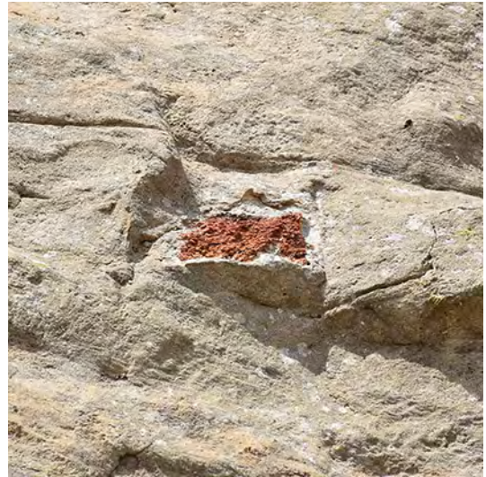
2.24: EVIDENCE OF BRICK BACKING
