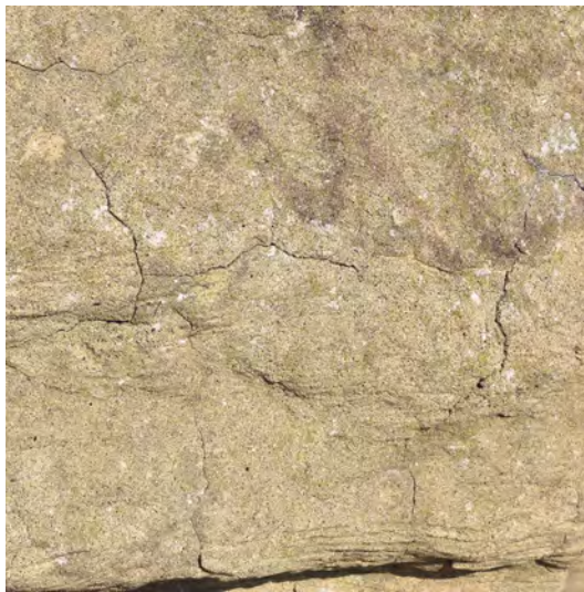
5.13: FINE SURFACE CRACKING (C12)
