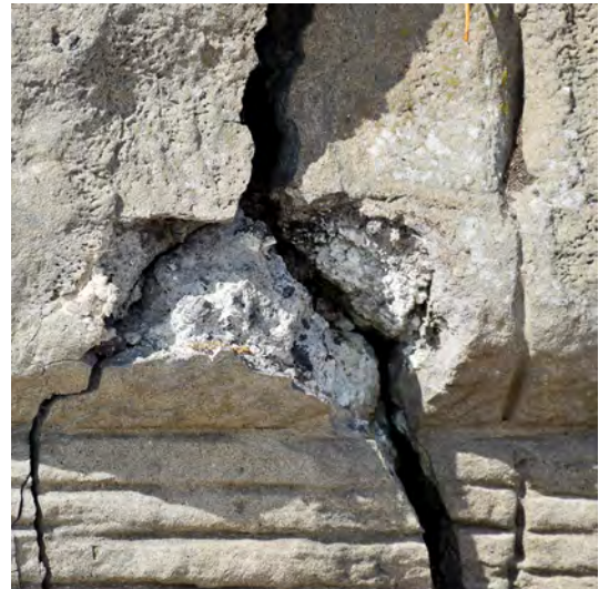
5.10: LOSS OF SURFACE AT FRACTURE (A32)
