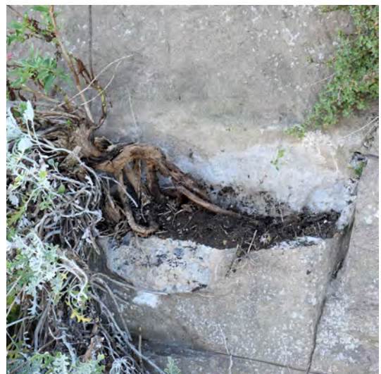
5.20: FAILURE DUE TO ROOT DAMAGE (B31)
