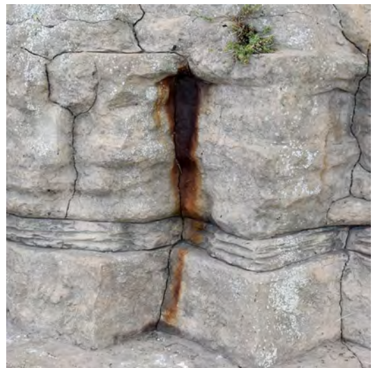
5.26: INTENSIVE METAL STAINING (A23)
