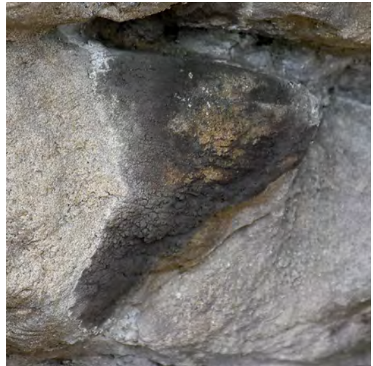
5.04: SULFATE CRUST (B01)
