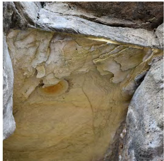
5.12: BREAK-DOWN & DELAMINATION OF STONE SLAB FORMING OVERHANG (B04B)
