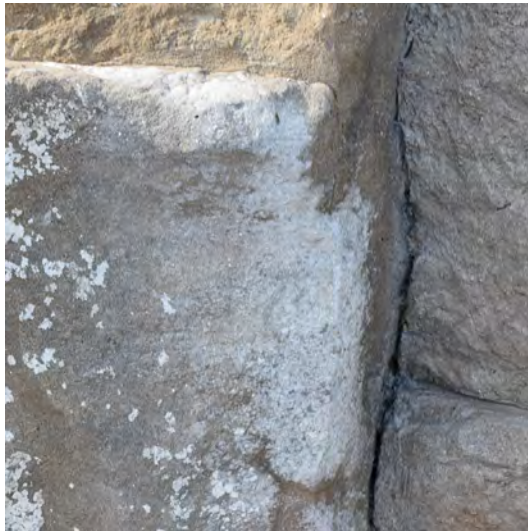
5.03: EFFLORESCENCE + LICHENS (B05)
