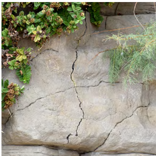
5.19: CRACKING DUE TO VEGETATION (A16)
