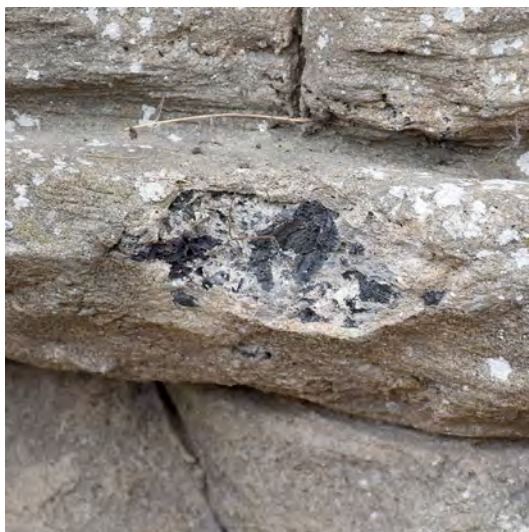
5.07: TYPICAL EXAMPLE OF MINOR LOSS OF PAR COATING (B01)
