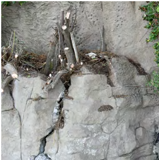
5.21: FRACTURE OF PLANT POCKET (A32)
