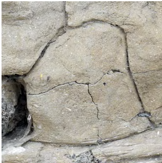
5.17: CRACKING — CHEMICAL AGENTS (A01)
