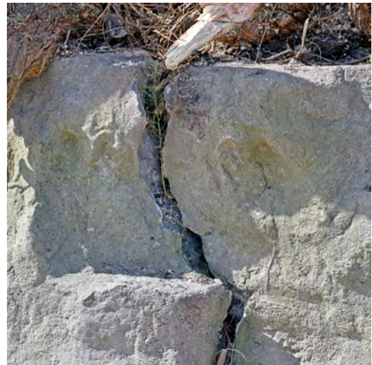
5.22: FRACTURE + DISPLACEMENT (A34)
