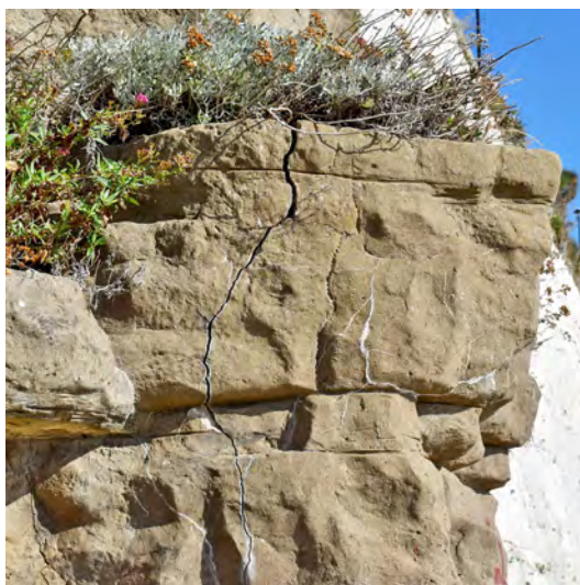
5.15: MAJOR FRACTURE (B22)
