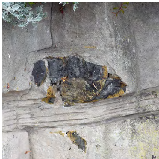
5.15: DAMAGE TO COATING & BACKING DUE TO VEHICULAR IMPACT (B08)
