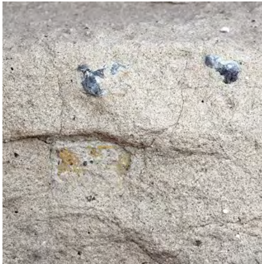
5.07: LIGHT EROSION & MINOR LOSS (C12)
