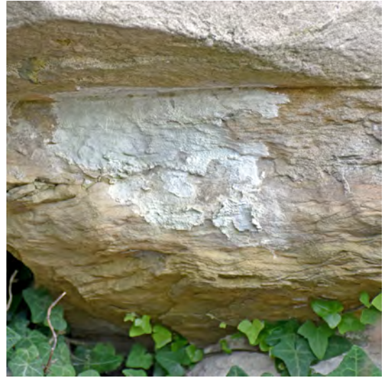
5.04: SURFACE EFFLORESCENCE (C11)
