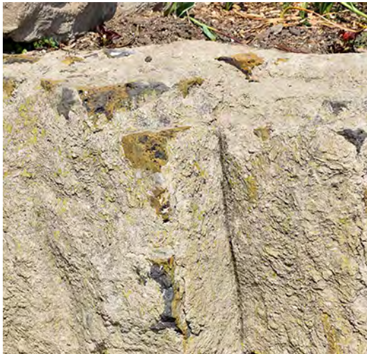
2.17: EROSION EXPOSES BRICKWORK
