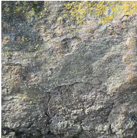
5.13: SCOURING DUE TO ORIENTATION (A05)
