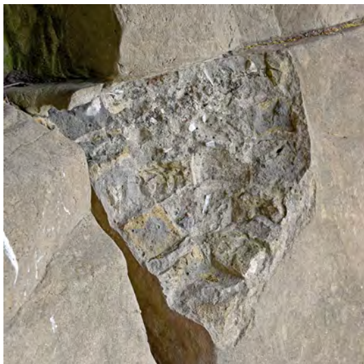
5.11: LOSS OF SURFACE LEAVING COATING & BACKING VULNERABLE TO WATER (C01)
