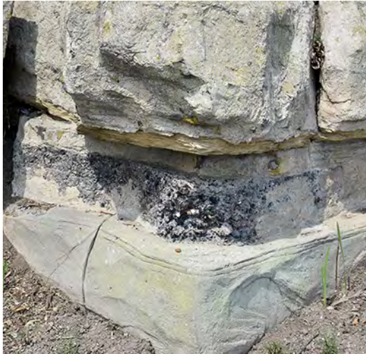
2.15: CONCRETE EXPOSED BY EROSION
