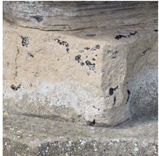
5.08: PITTING & GRANULATION (B05)
