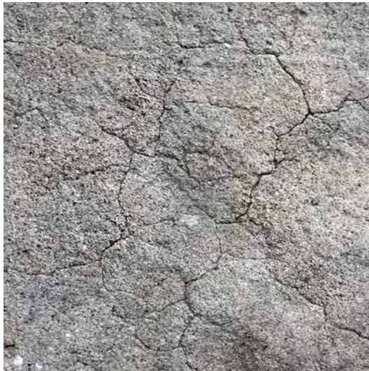
5.17: FINE SURFACE CRACKING (A16)
