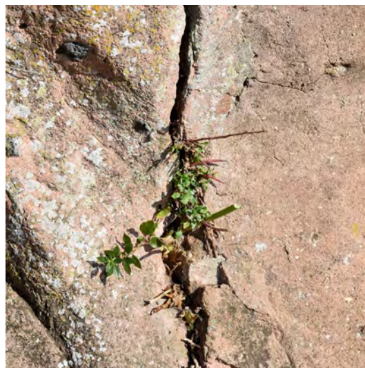
5.22: WOODY VEGETATION SELF-SOWN IN OPEN FRACTURE (B15)
