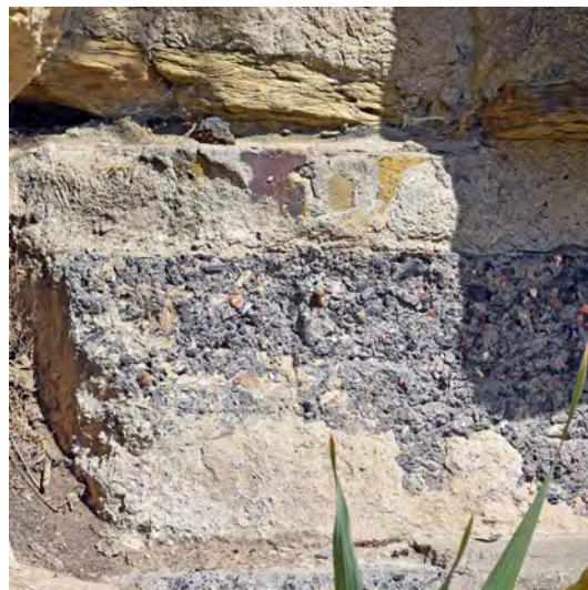
5.12: LOSS OF COATING DUE TO SALTS & PREFERENTIAL WEATHERING (D02)
