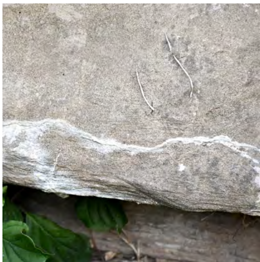
5.21: HORIZONTAL V SULFATE ATTACK AT BASE OF PLANT POCKET(C15)
