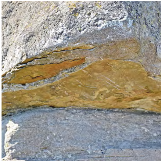
5.09: UNDERSIDE LOSS OF COATING (B13B)
