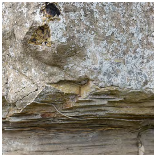
5.16: DELAMINATION TO UNDERSIDE OF STONE SLAB OVERHANG (B05)
