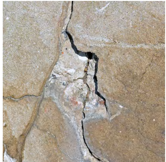
5.10: SURFACE LOSS & FRACTURE (C06A)
