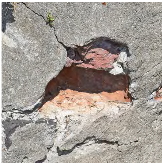
5.13: LOSS OF SURFACE LEAVING COATING VULNERABLE TO WATER (N37)
