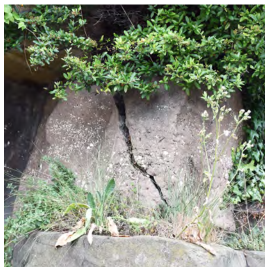
5.20: FRACTURE & DISPLACEMENT (N19)
