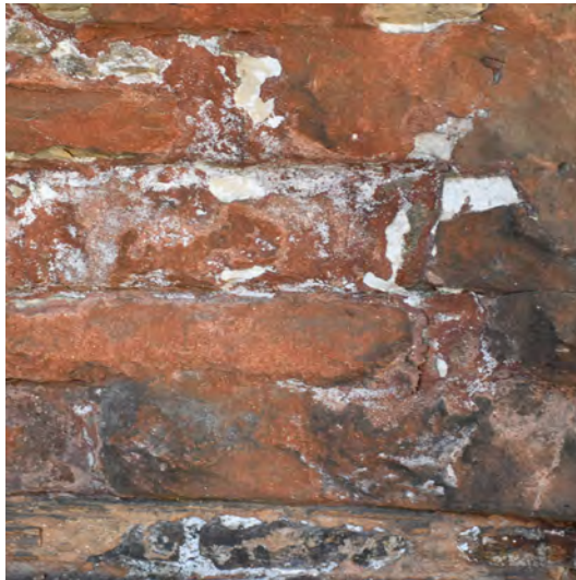
5.03: SURFACE EFFLORESCENCE (S08B)
