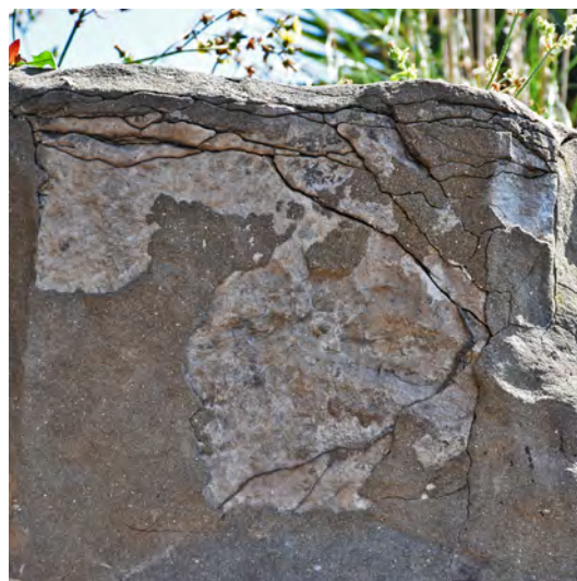
5.16: FROST DAMAGED CHALK (S08C)
