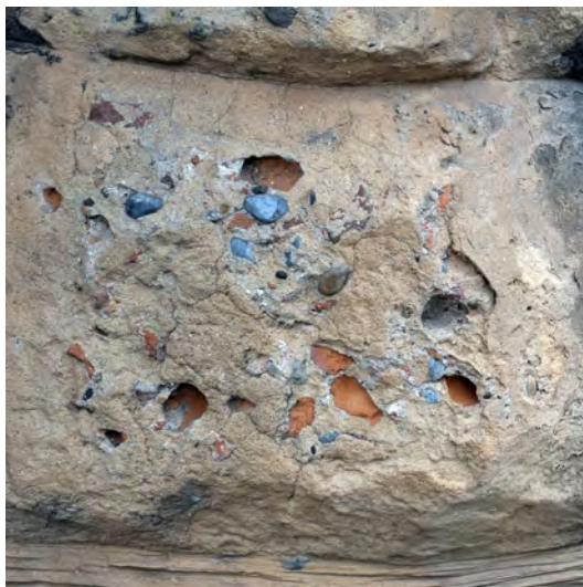
5.09: PITTING &amp; HOLLOWNESS (N09)
