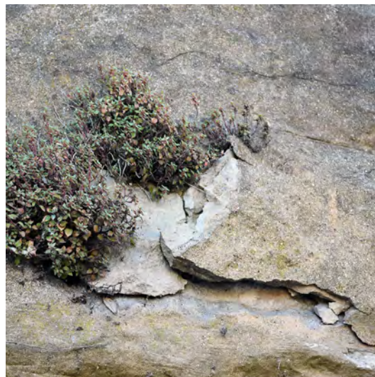
5.14: PARTIALLY DETACHED AREA OF COATING AT HIGH LEVEL (S09)
