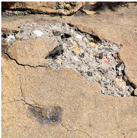
2.33: LOSS OF SURFACE EXPOSES ROUGH CONCRETE BACKING
