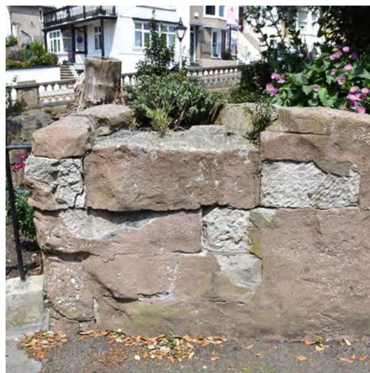
5.12: SURFACE LOSS — SHEARING FROM CHALK BLOCKS DUE TO FROST (S01)
