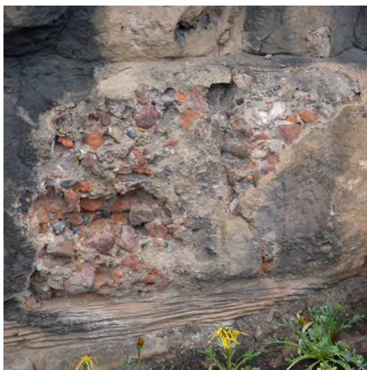
5.11: SURFACE LOSS DUE — PREFERENTIAL WEATHERING DUE TO ORIENTATION (N09)
