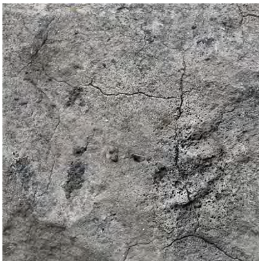
5.17: FINE SURFACE CRACKING (N03)
