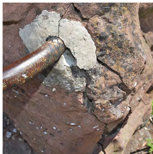
5.22: FRACTURE — EMBEDDED IRON (S04)
