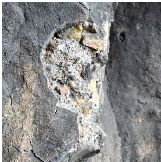
5.15: IMPACT DAMAGE (N16)
