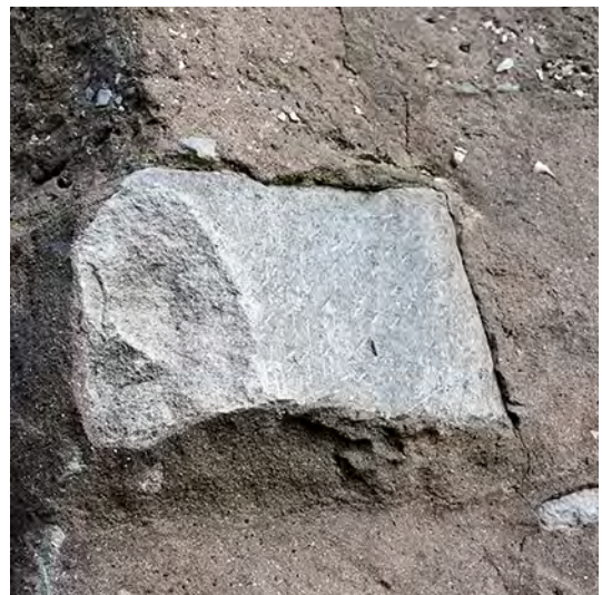
2.34: GRANITE WITHIN BACKING REVEALED BY LOSS OF SURFACE
