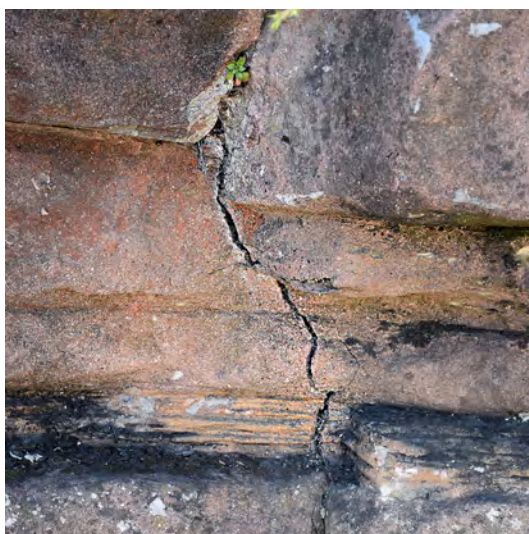
5.19: MAJOR FRACTURE (S07)
