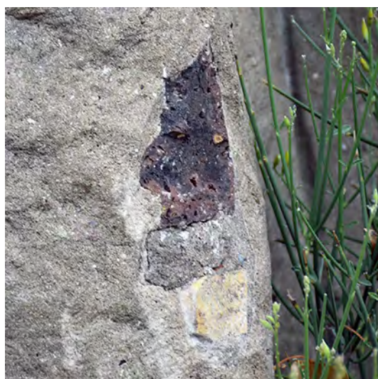
5.07: LOSS OF SURFACE DUE TO IMPACT
