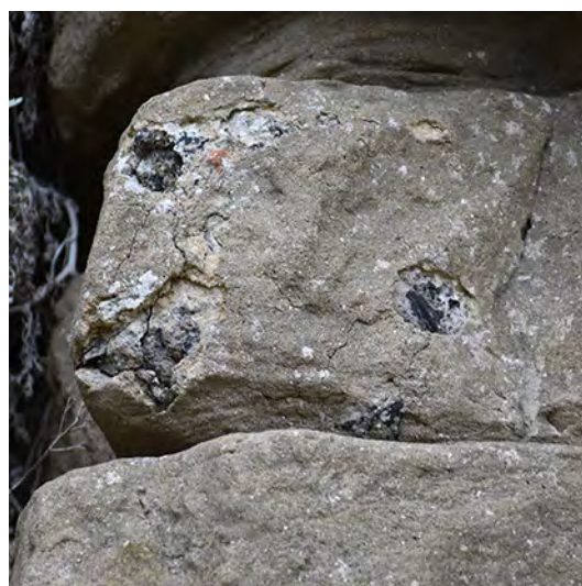
5.08: EVIDENCE OF FROST DAMAGE
