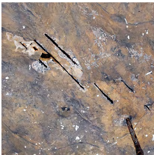
5.09: LOSS OF COVER & CORROSION OF REINFORCEMENT (UNDERSIDE OF BRIDGE)
