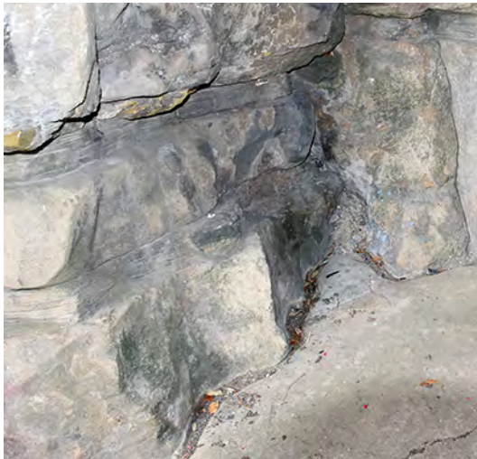
5.03: AIRBORNE DIRT BENEATH ARCH
