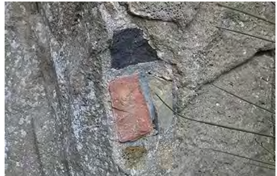
2.12: BRICK BACKING EXPOSED WHERE SURFACE HAS DETACHED
