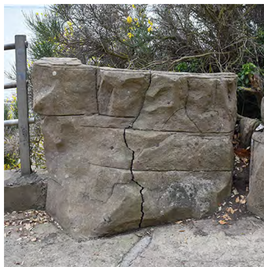
5.10: FULL HEIGHT FRACTURE TO FINAL BLOCK OF ROCKWORK (SOUTH SIDE)
