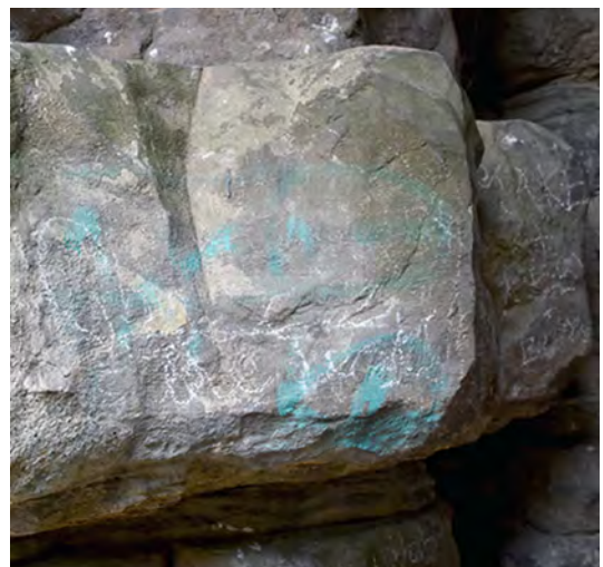
5.06: GRAFFITI (CHALK & SPRAY PAINT)
