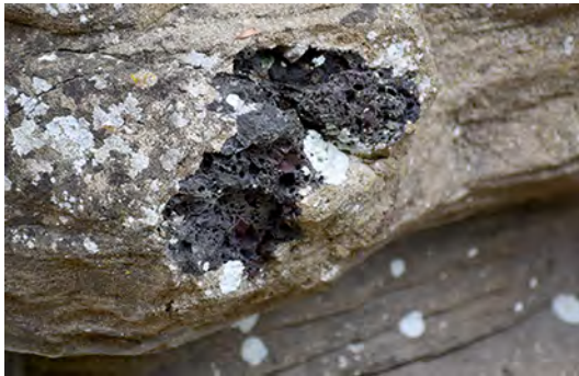
2.11: LOSS OF SURFACE EXPOSES ROUGH CONCRETE BACKING
