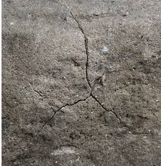
5.11: SURFACE CRACKING (WEATHERED EDGES SUGGEST HISTORIC)
