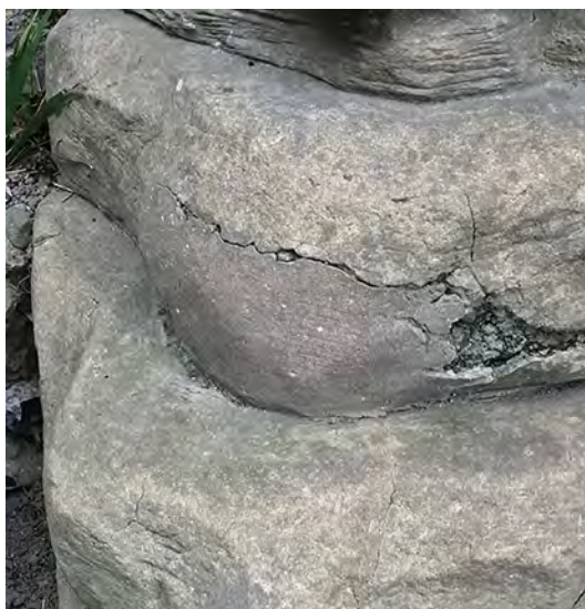
5.13: ILL-MATCHED RENDER REPAIR (TEXTURE & COLOUR) — FAILING
