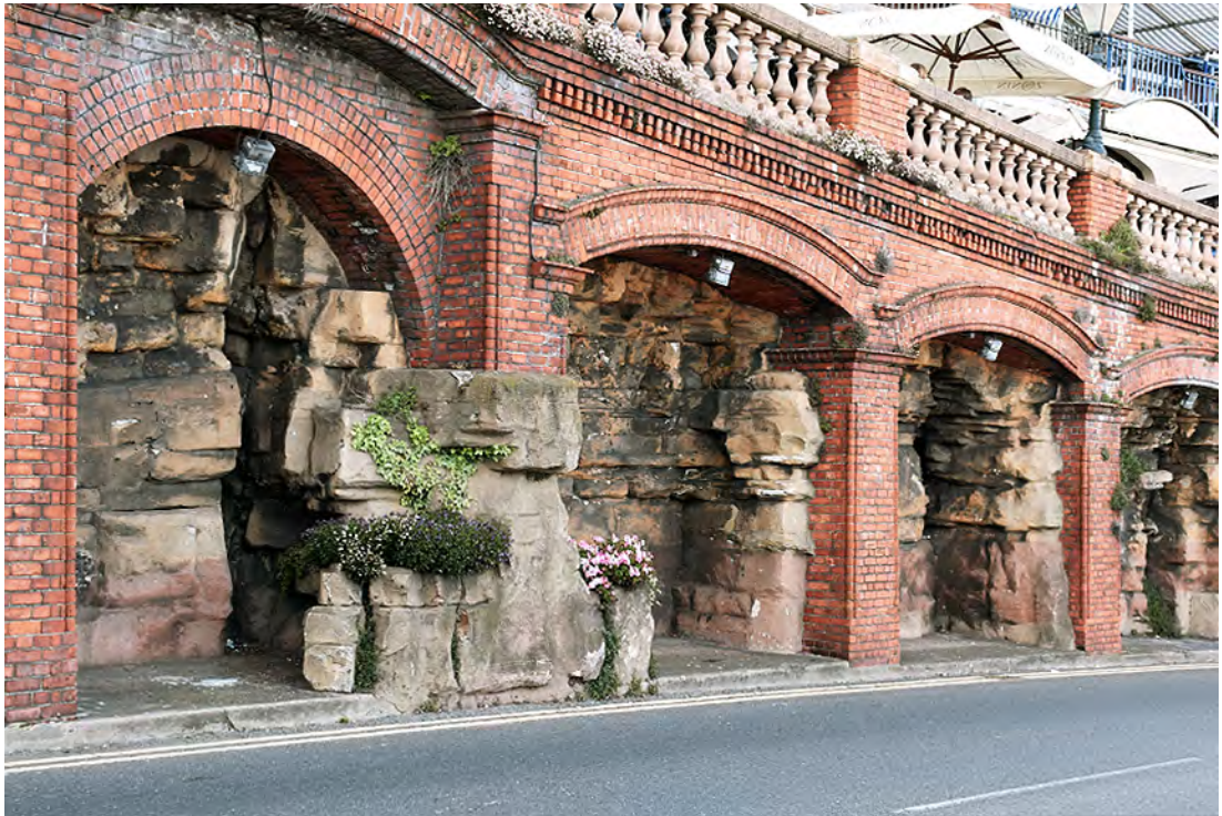
2.08: PAR ROCKWORK WITHIN FRAMEWORK OF BRICK ARCADE SHOWING LACK OF PAVEMENT & ROCKWORK BREAKING FORWARD ACROSS BAYS 20 & 21
