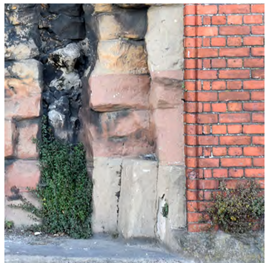
3.04: PARIETARIA JUDAICA, GROWING IN FISSURES & MORTAR JOINTS (BAY 23)
