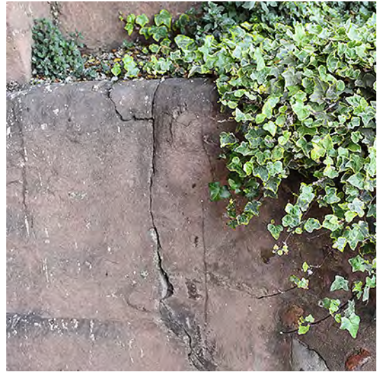
5.13: VERTICAL FRACTURE OF PLANT POCKET DUE TO WOODY GROWTH
