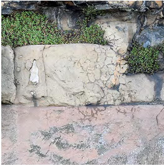
5.12: CRAZED PATTERN OF CRACKING INDICATES SURFACE BREAKDOWN
