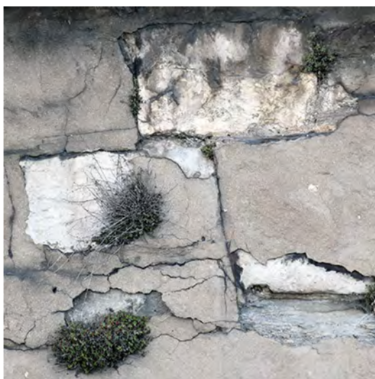
5.10: LOSS OF COATING FROM CHALK
