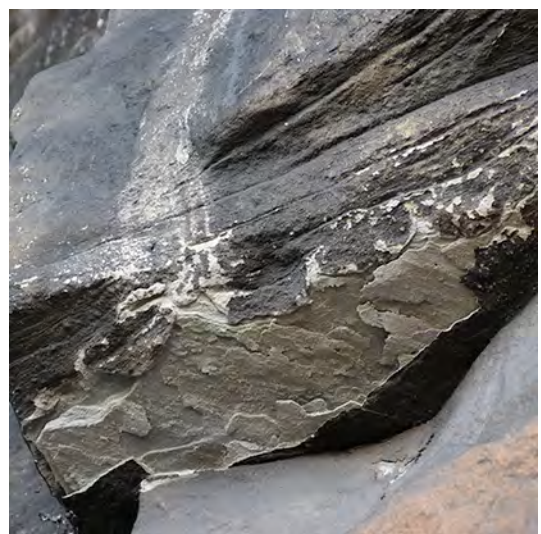
5.11: TYPICAL UNDERSIDE LOSS
