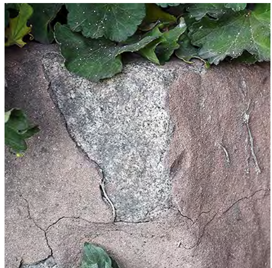
5.09: COATING LOSS (STONE BACKING)
