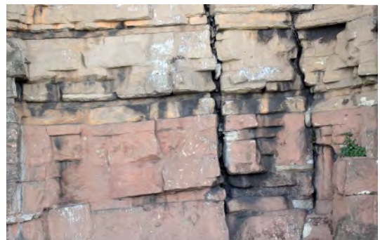
2.12: CLEFTS, FISSURES & COLOUR (BAY 19)
