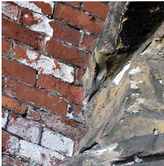
5.05: SALTS INDICATE WATER PENETRATION OF BRICKWORK FROM ABOVE
