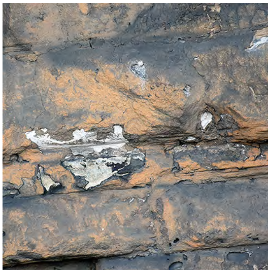
5.08: TYPICAL LOSS OF COATING
